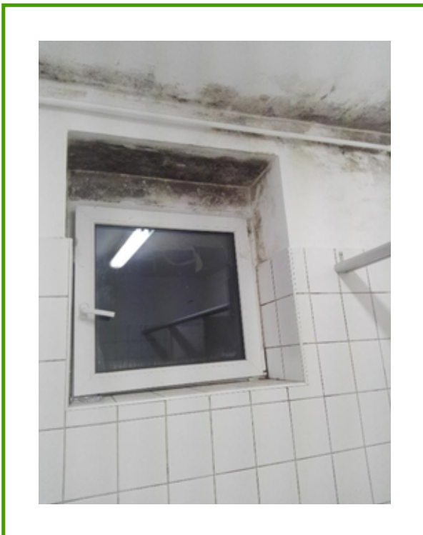
Figure 17: Mould growth after window change, due to thermal bridges and insufficient ventilation 47
